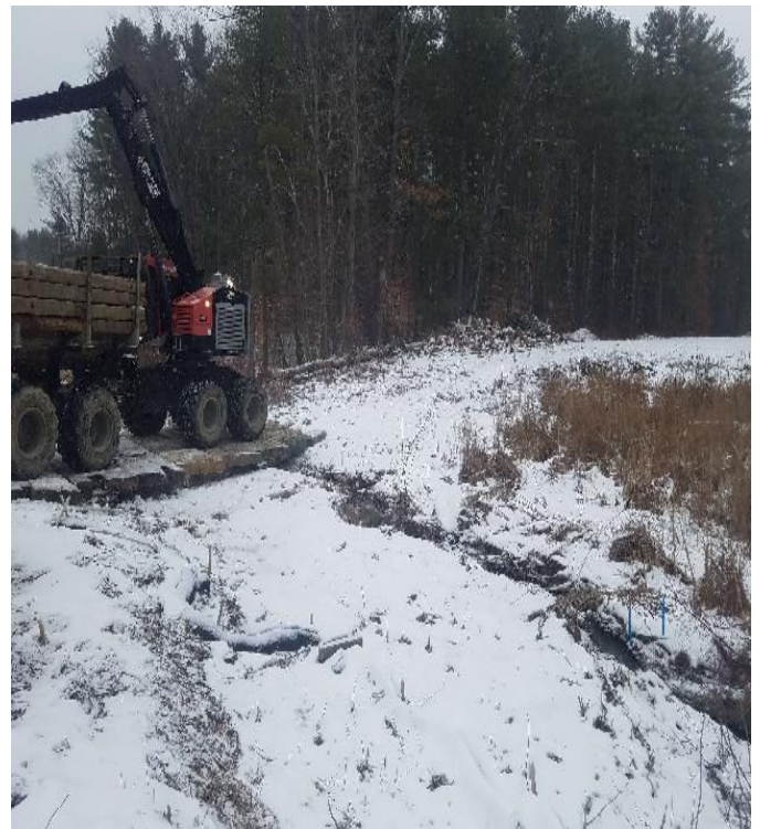
Fig 14: Crew beginning to build matted access road from Str. 112 to Str. 114. Viewing northeast. (02-18-20).
