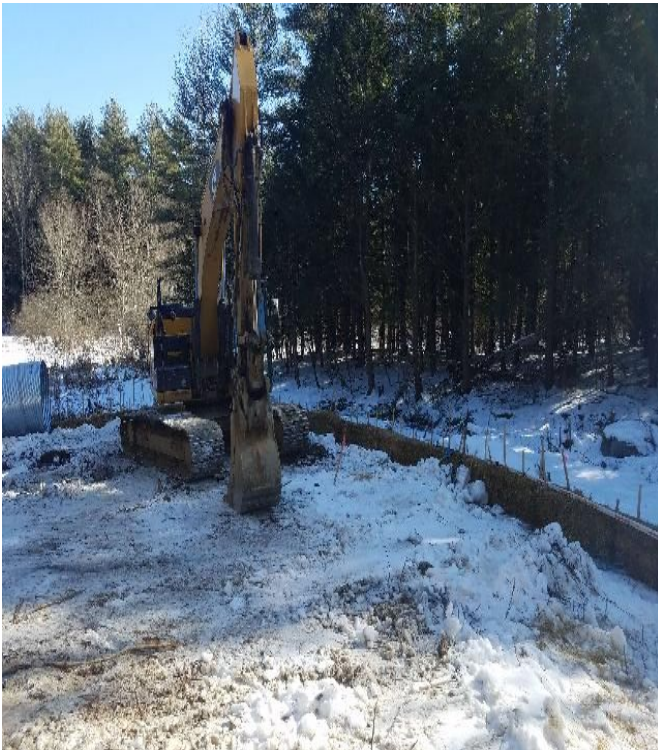
Fig 7: BMPs installed around the perimeter of the work area at Str. 68. Viewing east. (02-14-20).
